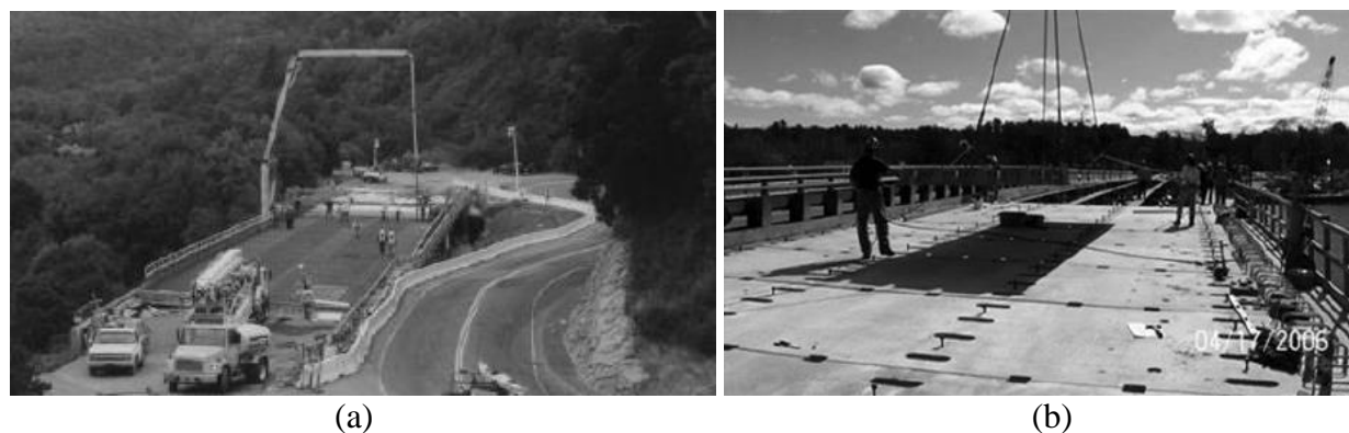
Fig. 17. Deck construction (Shen 2014): (a) cast in place; (b) assembly of precast panels
